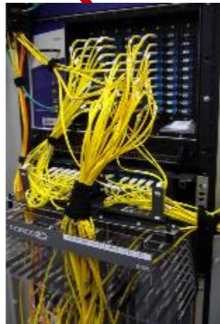
Campus Optical Switch
