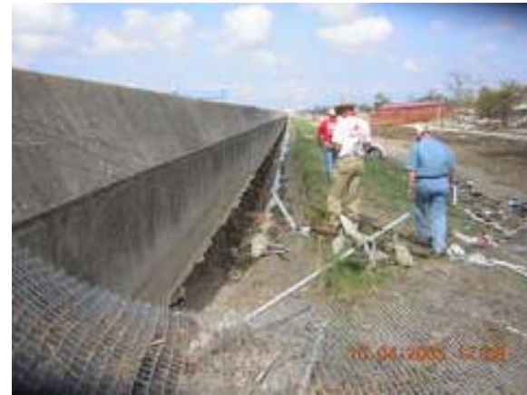
Engineers examine the scoured trench behind the concrete floodwall next to the catastrophic levee breach at the west end of the Lower Ninth Ward of New Orleans. Credit: Rune Storesund
